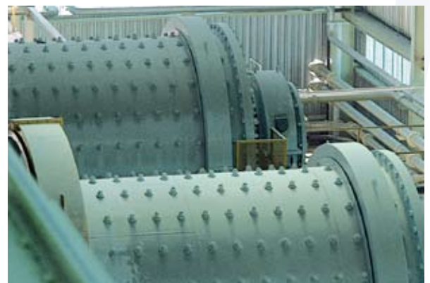
Scrubber at Finch Diamond Mine, South Africa (4 m x 7,4 m dia.)
